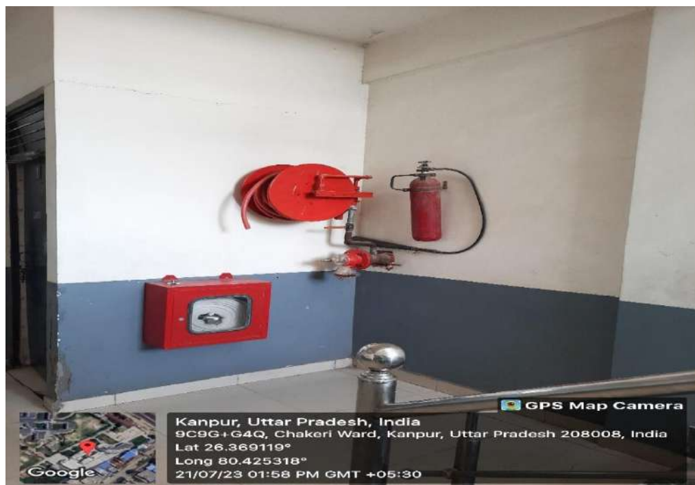
Fire safety System 1 (Academic Block)
