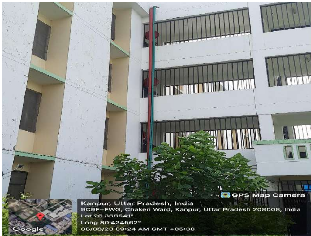
Fire Safety System 4 (Girls Hostel)
