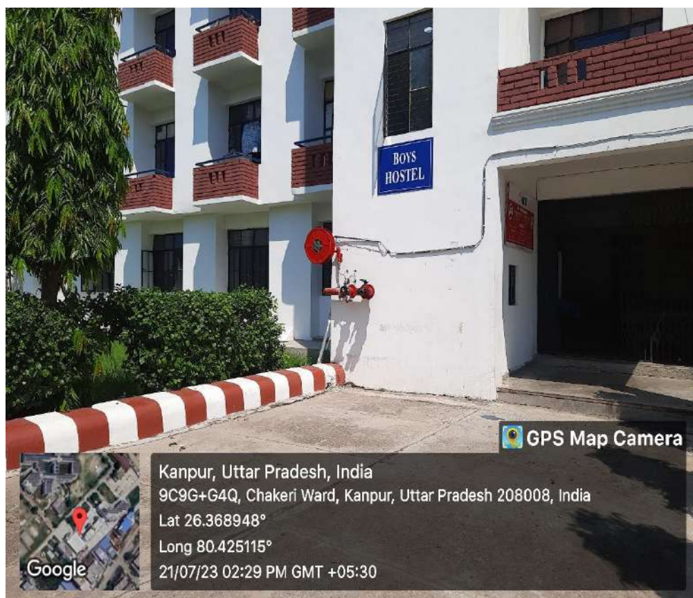
Fire Safety System 3 (Boys Hostel)
