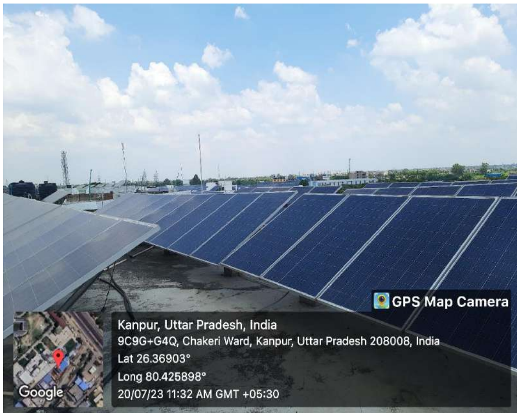
Solar Power Plant 3
