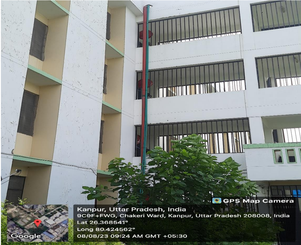
Fire Safety System 4 (Girls Hostel)
