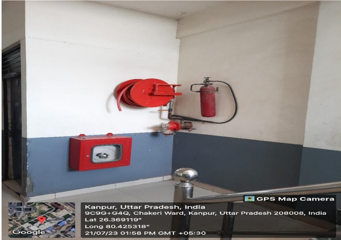
Fire safety System 1 (Academic Block)
