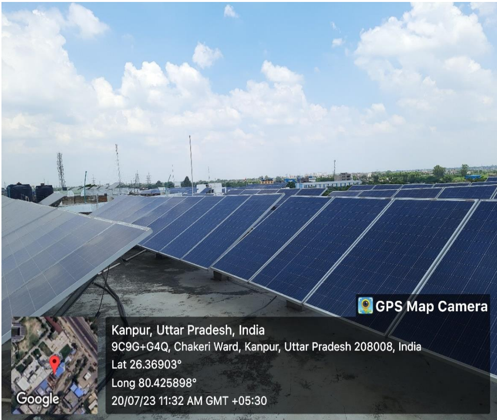
Solar Power Plant 3
