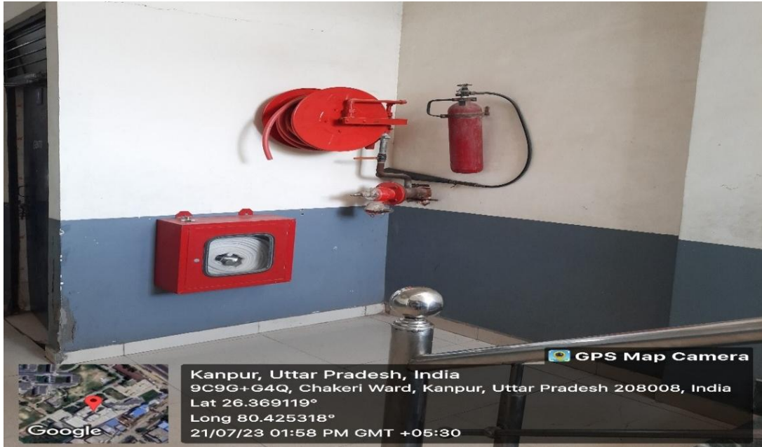
Fire safety System 1 (Academic Block)
