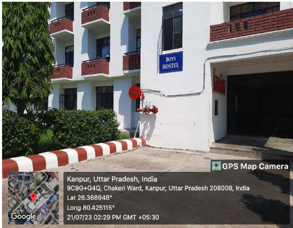
Fire Safety System 3 (Boys Hostel)
