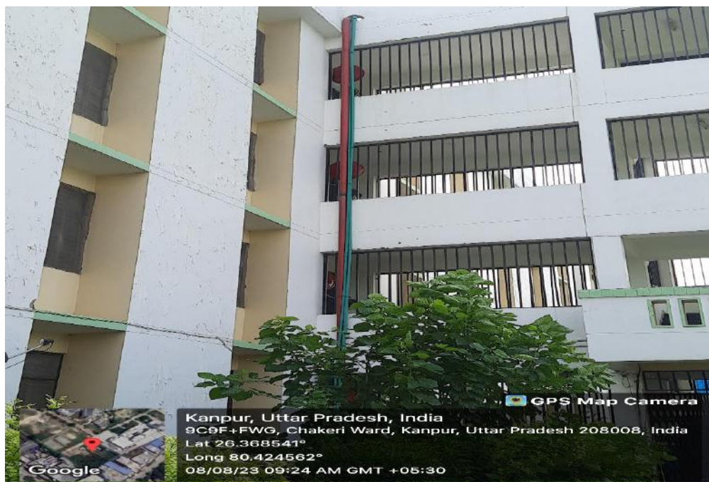
Fire Safety System 4 (Girls Hostel)
