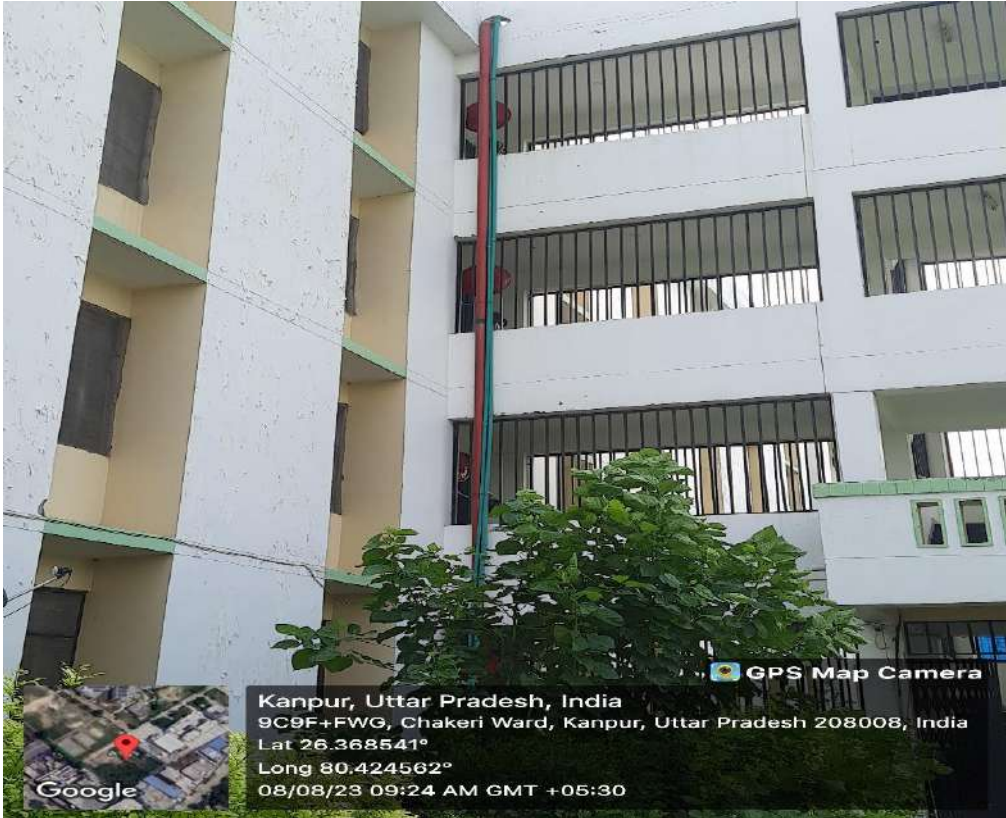
Fire Safety System 4 (Girls Hostel)
