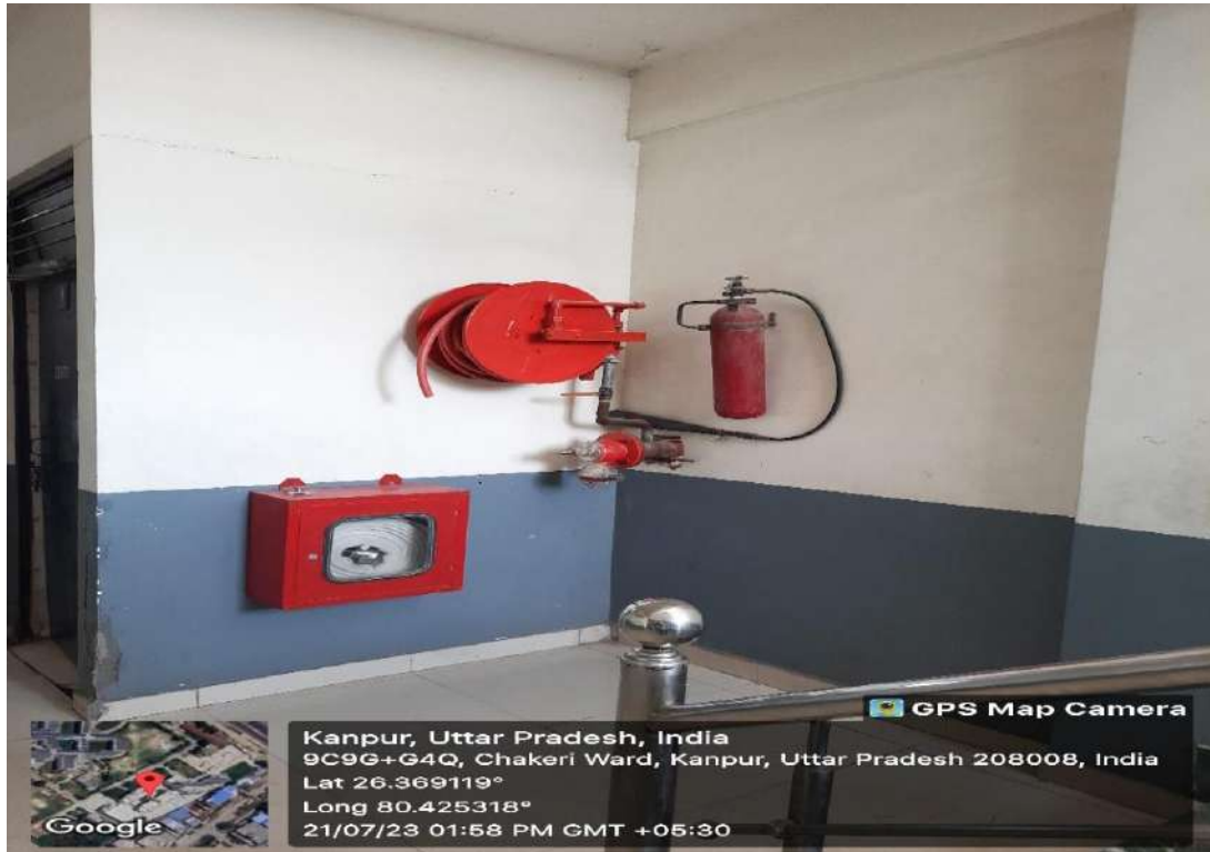
Fire safety System 1 (Academic Block)
