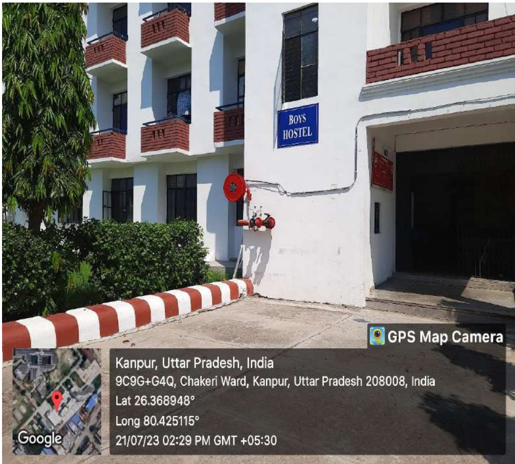
Fire Safety System 3 (Boys Hostel)
