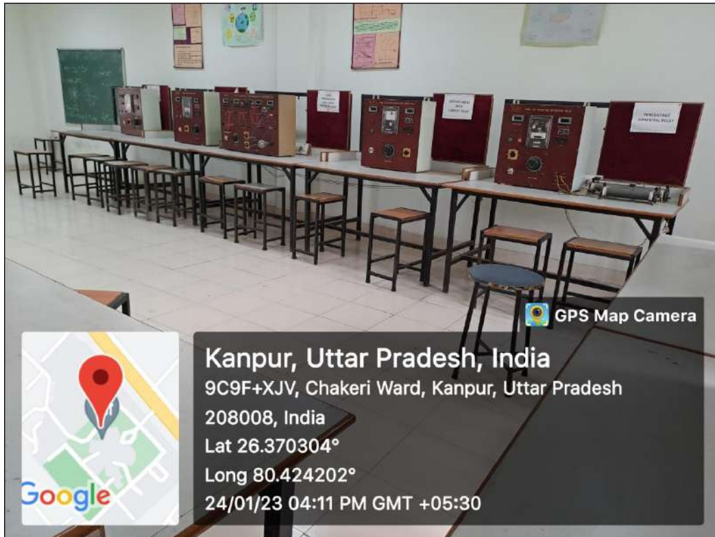
Lab 57: Power System Lab
