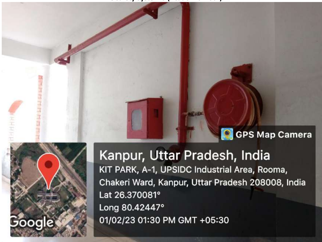
Fire safety System 4 (Academic Block)
