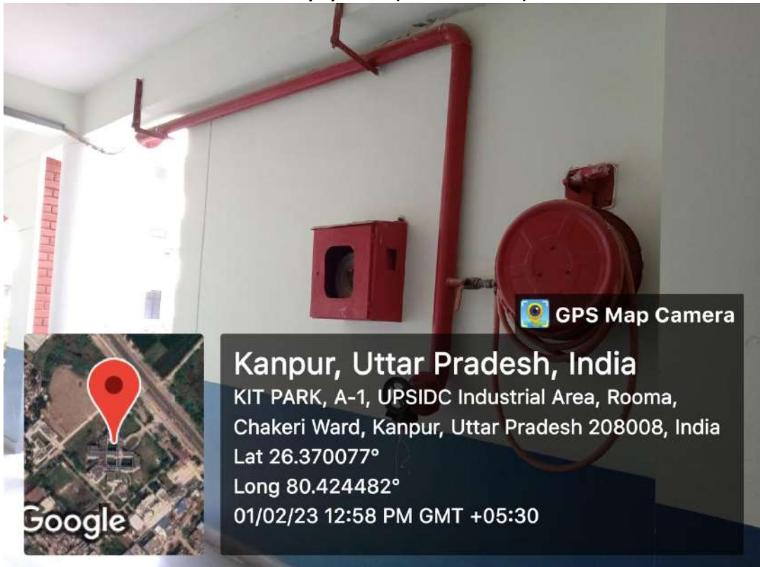
Fire safety System 2 (Academic Block)
