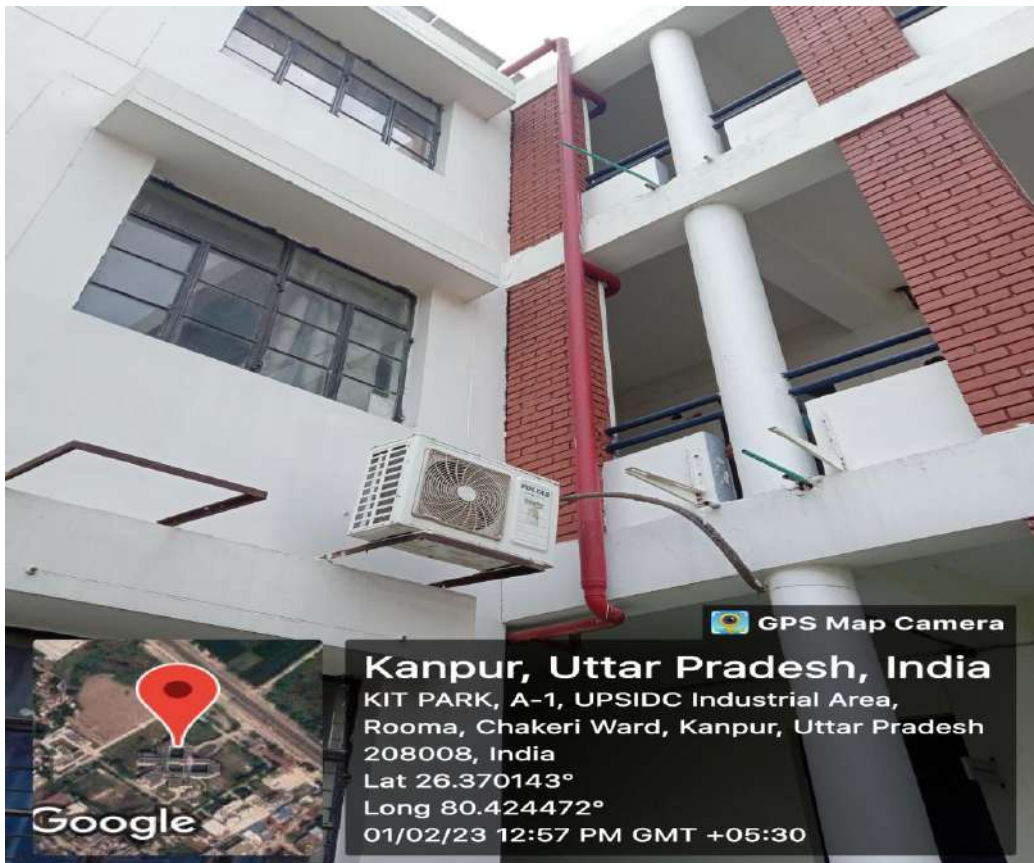
Fire safety System 3 (Academic Block)
