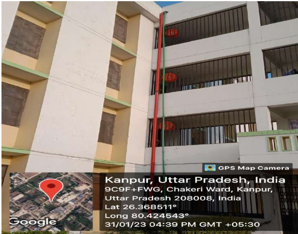
Fire Safety System 7 (Girls Hostel)
