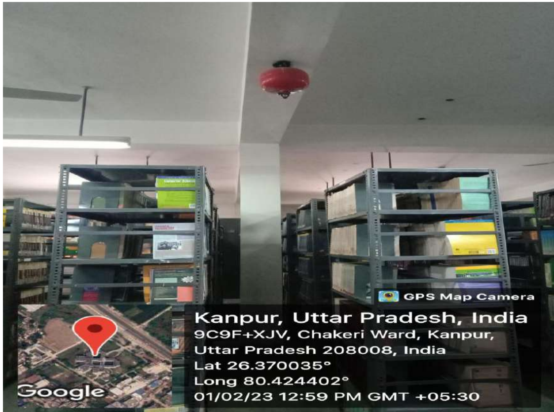
Fire safety System 5 (Library)
